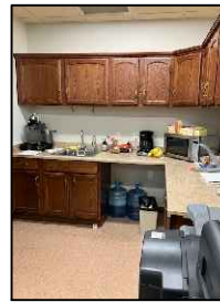
D. Cabinets and counter to be replaced.
