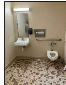
F. Sink, toilet and fixtures to be removed.
