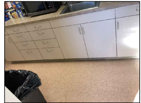
I. Flooring to be replaced.
