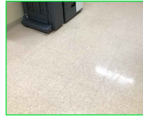
D. Flooring to be replaced.
